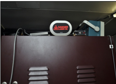
Figure 3-5: Lighted laser warning sign posted at the entrance
